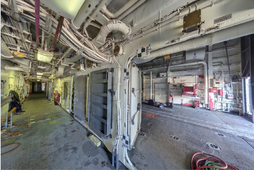
The last image is a bubbleview of USS Samuel B. Roberts (FFG-58) Hanger deck, captured and processed with a Z+F scanner using automation assisted processing. It is ready to support ship lifecycle applications.
