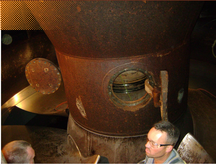
Turbine shaft casing with access hatches
